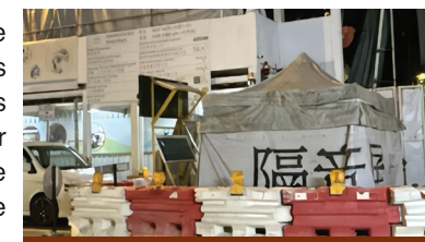
可移動隔音屏障 Movable noise barriers
